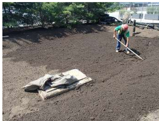
An example of a bioinfiltration basin installation
